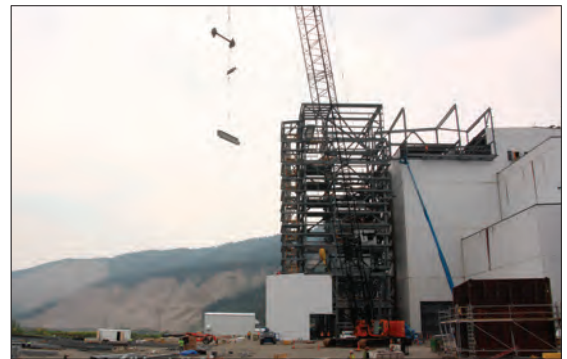
The Selective Catalytic Reduction (SCR) addition is shown under construction. This is a new addition to Unit 2 and will house the new environmental controls. Much of the equipment has already been installed, since the easiest way to install it is to erect the building around it. Photo by Tina Graham
