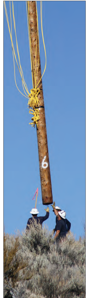
A line crew guides pole six from the helicopter into its receiving hole, where it is plumbed and stabilized before backfilling.
