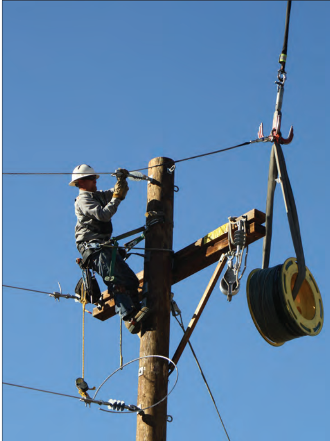
A helicopter hovers with a weighted spool above Rob Azevedo while he ties a primary distribution line off at the last pole.
