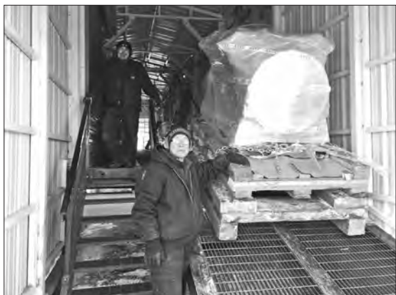
Will Peterson and Edward Twitchell helped roll the engine up into the module the old-school way, using chains, steel pipes, a come-along, great teamwork and brute strength.
