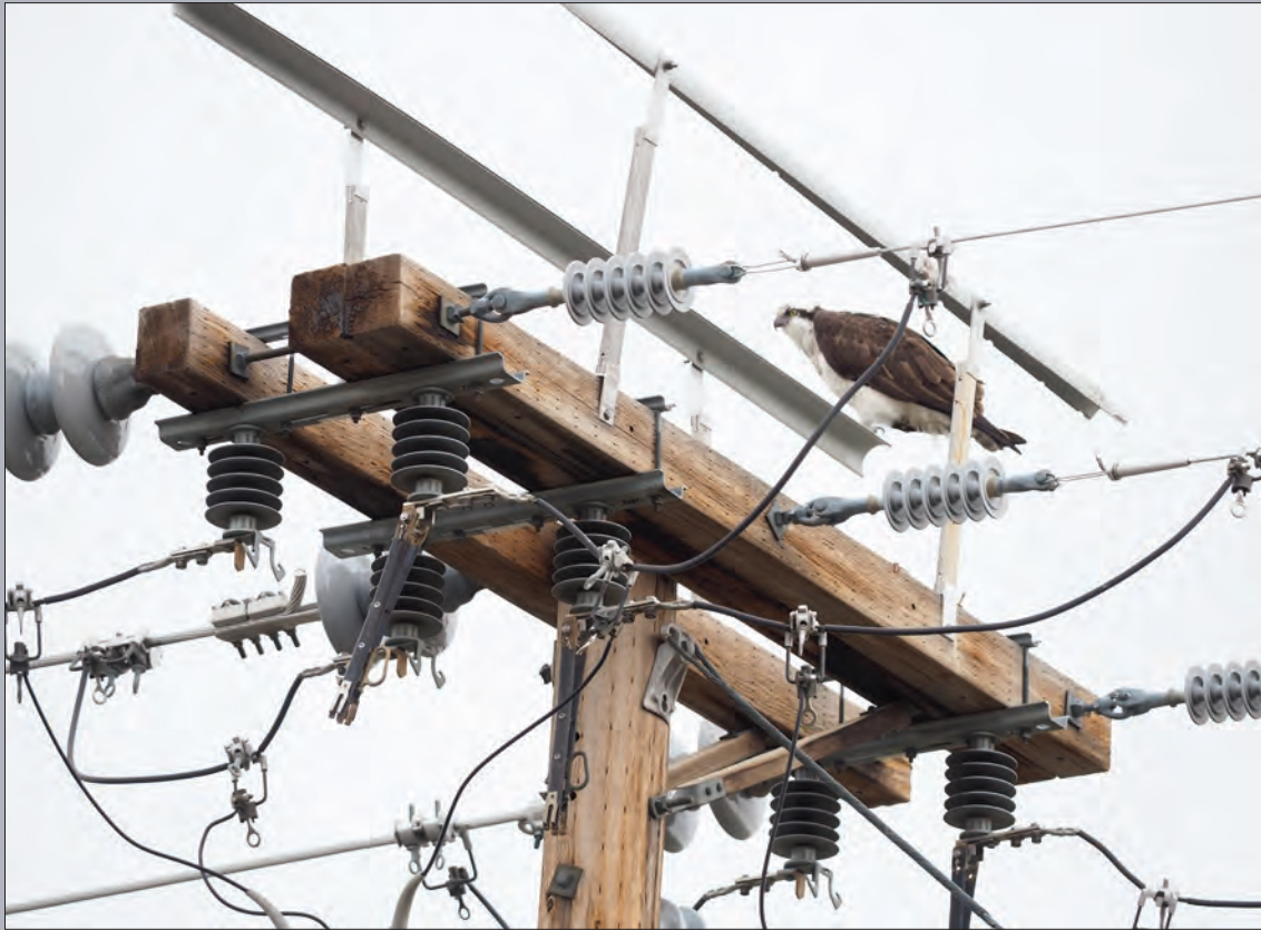
Perches installed on many CEC power poles provide high spaces for birds to nest safely.
