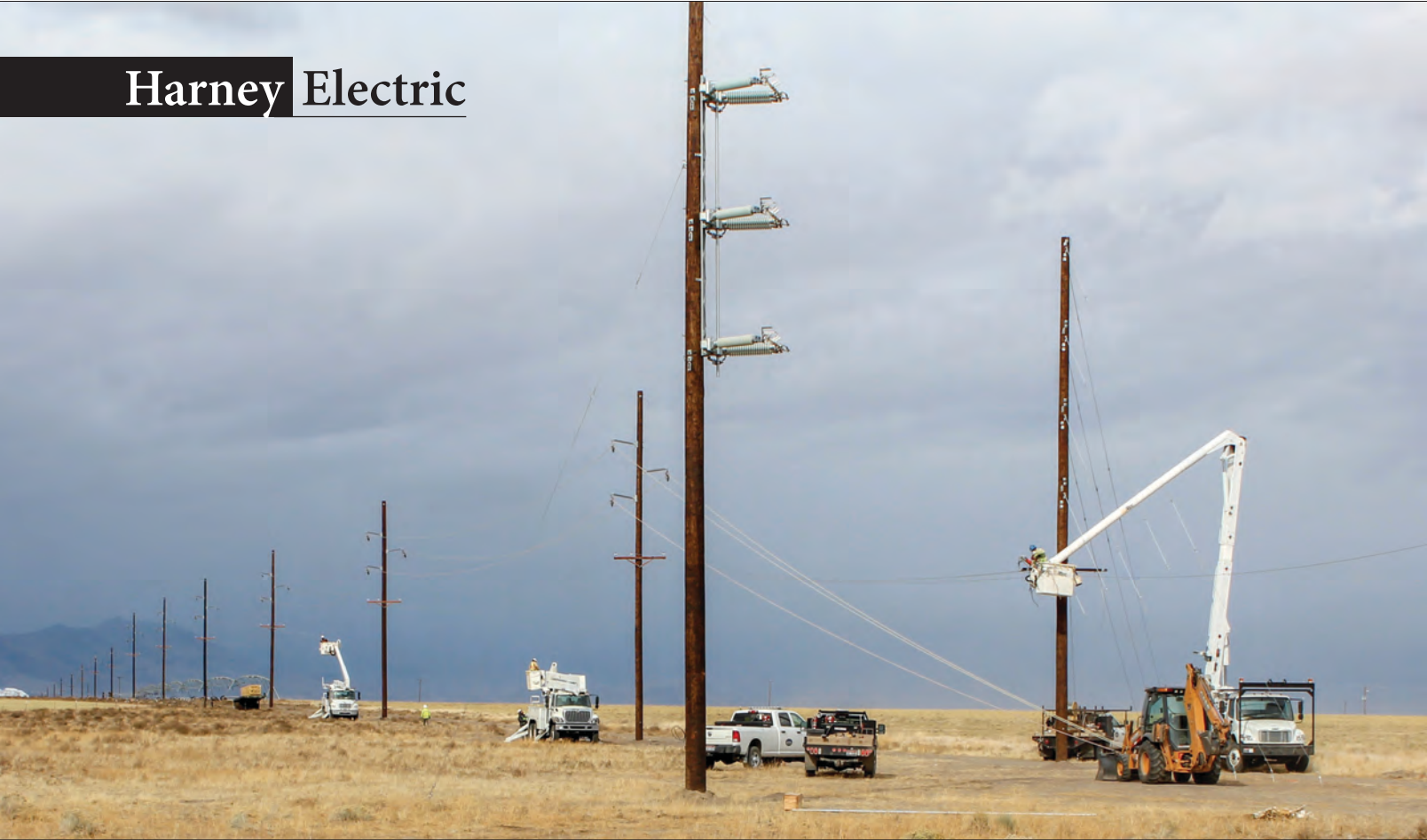
Crews from Probst work on power lines near Fields Substation as ominous weather approaches.
