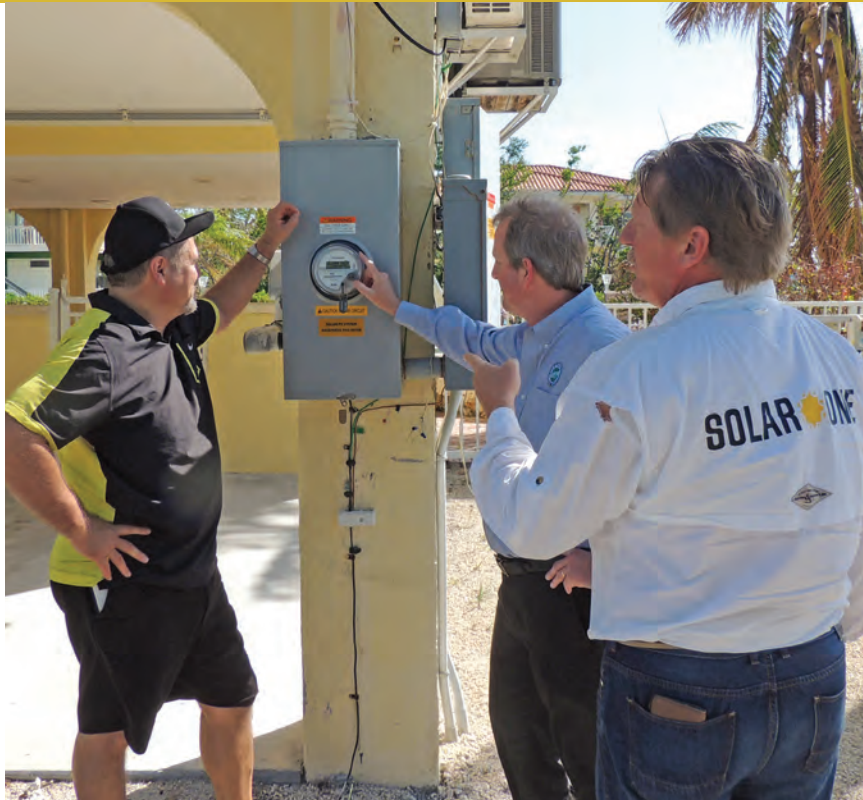
From left, FKEC Member Dr. John Massimilian, FKEC Member Service Representative T.J. Patterson and Solar One Owner Ray Johnson, PE discuss the solar arrays bi-directional meter. This meter allows a home to produce its own energy while also drawing electricity from FKEC.
