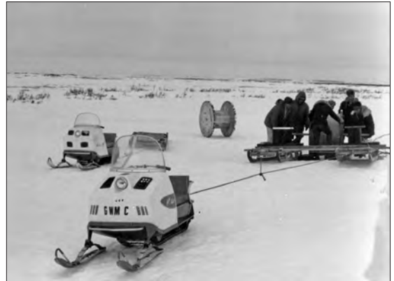
Village residents eager to have electric power helped install distribution and generation facilities in the late 60s and mid 70s.
