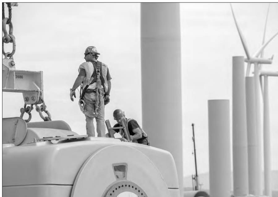
"We're providing jobs in the area," Ormand says. "On a dollar-to-dollar basis, there is more return to the local economy on the small projects than the larger projects." Here, a construction crew sets a spreader bar used by a crane to lift the generator and gearbox housing onto the top tower.
