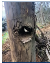
Crews were cautious after pulling this pole up with a gas line running through it.
