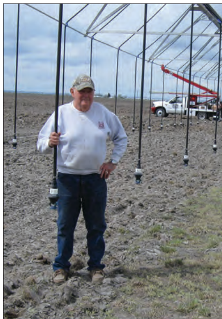
Earl Barber shows the height of the new sprinkler package on his property in Burns.
