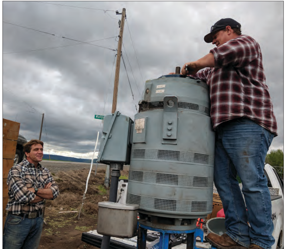
Cove farmer Marc De Lint, left, discusses the benefits of adding variable frequency drives to irrigation pumps with Gunnar Rolf, a technician with Roman's Precision Irrigation. Gunnar was getting the motor ready to run before hooking up the VFD.
