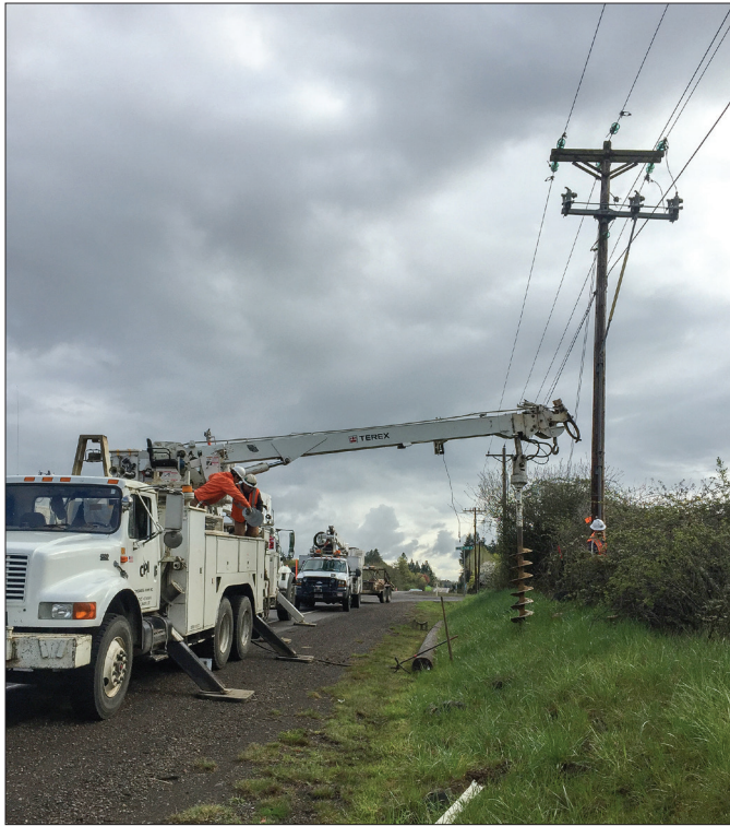
CPI crews use a digger truck to dig a hole and place a new pole.
