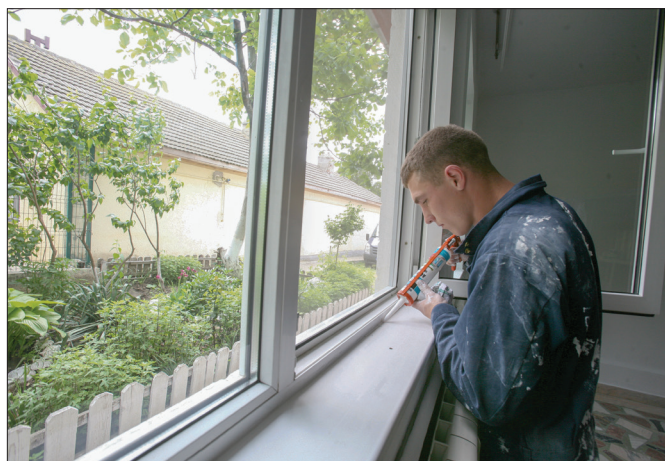
Sealing air leaks is critical to keeping the interior cooler than the exterior.
