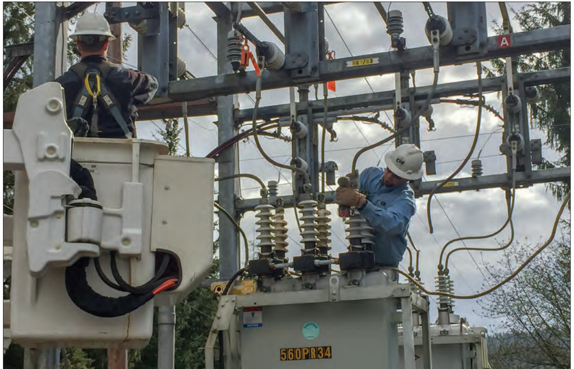
Crews from Consumers Power Inc. in Philomath, Oregon, replace insulators at a substation near the Oregon Coast.
