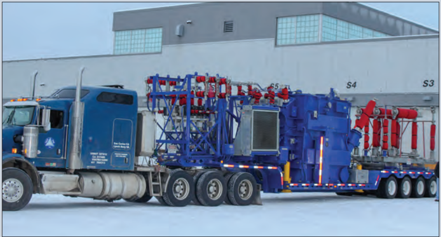
After a 10-day, 3,500-mile road trip, a new 20 MVA mobile substation from California arrived at Golden Valley Electric Cooperative in Fairbanks, Alaska, on December 24, 2017.
