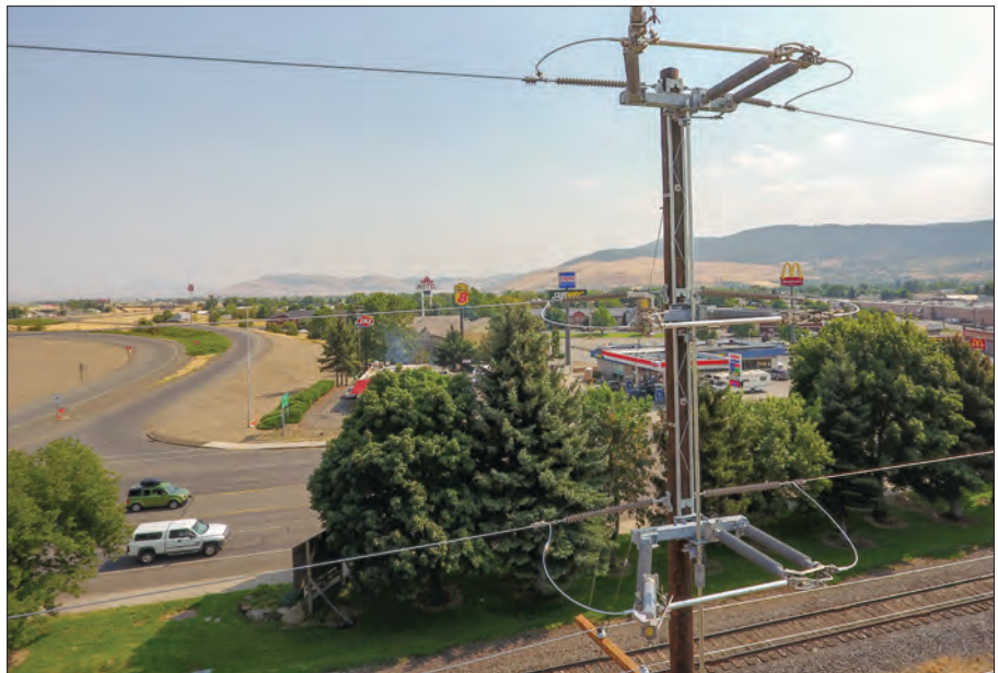
This photo taken from a drone shows the condition of a pole and its equipment in the La Grande district.
