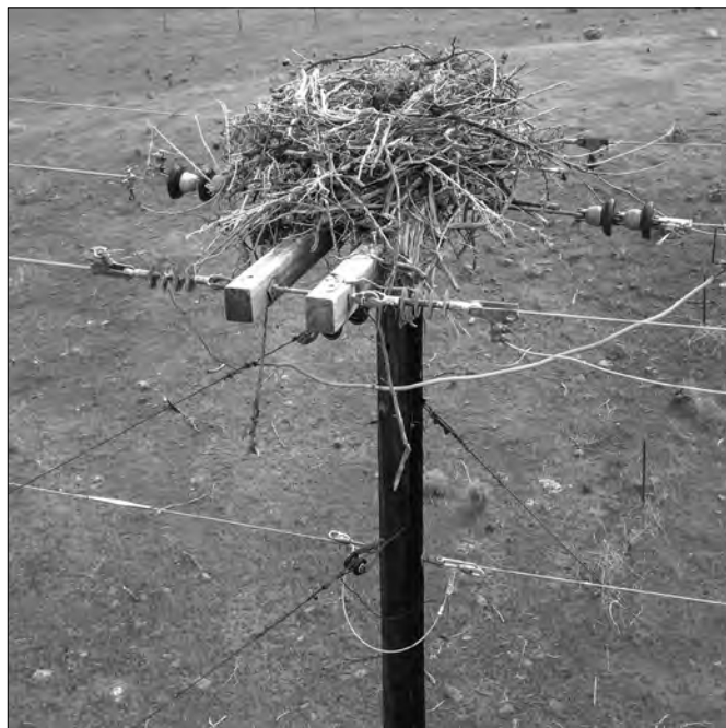
Osprey nests can create power outages. Platforms, such as this one along the Deschutes River near Maupin, help keep the system reliable.
