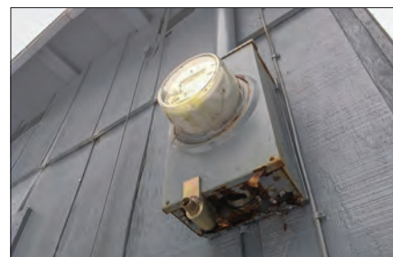
A rusted meter base is a safety hazard and should be repaired by the homeowner.
