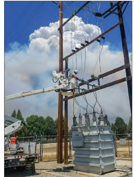
Lineman Scott Davies isolates the AEC feeder from the switch station so the Lake Hemet Substation can be back fed from the temporary generator.
