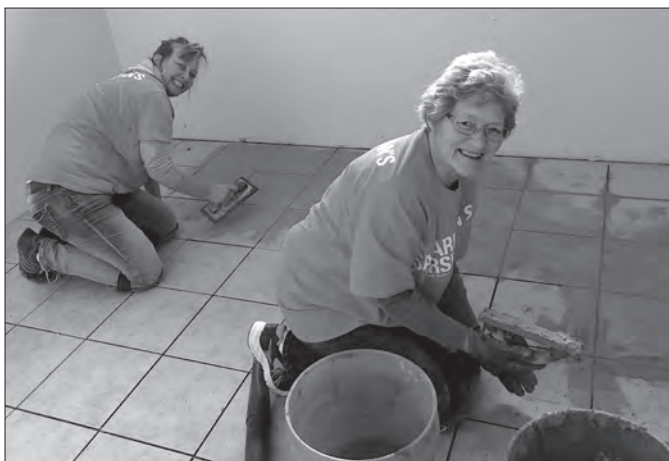
Jennifer Simcoe and Pat Stiles lay tile during a disaster recovery trip to Houston. They were among 13 parishioners from the small church in Paul to volunteer through Samaritan’s Purse.
