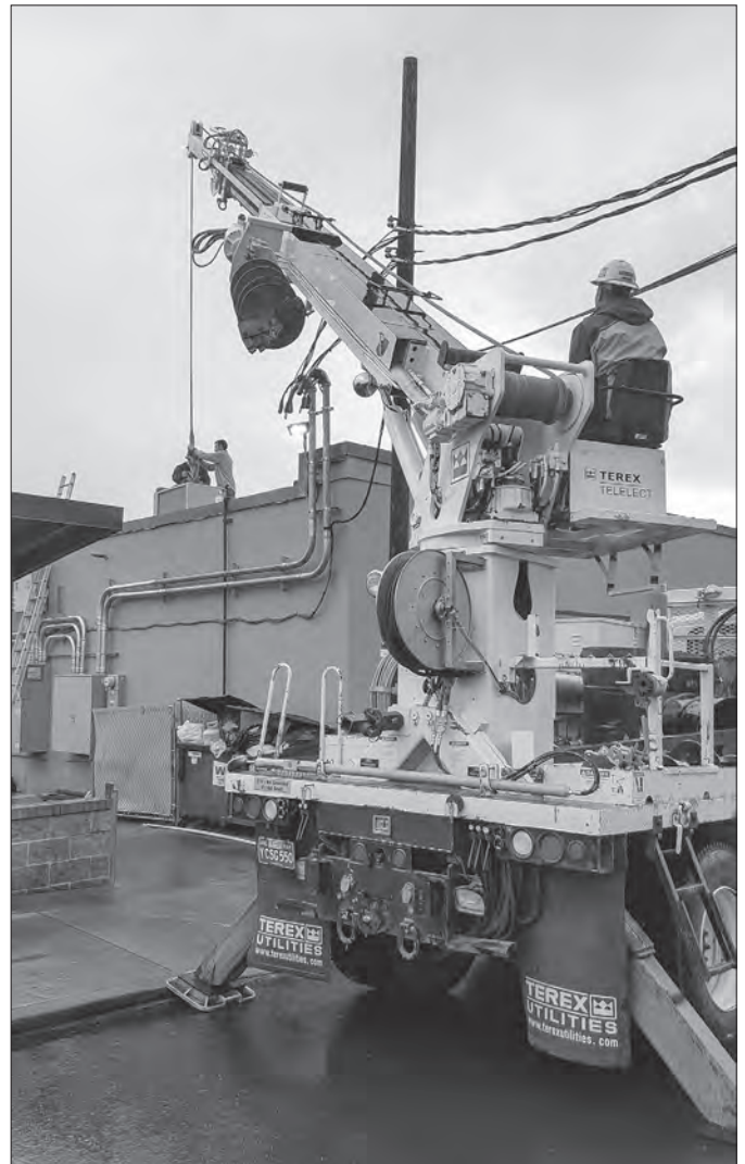
WOEC workers lift a refrigeration compressor onto the roof of the R&S Market in Vernonia.
