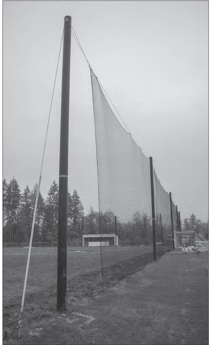
The Vernonia School District received help from WOEC to set and anchor poles at its new baseball and softball fields.
