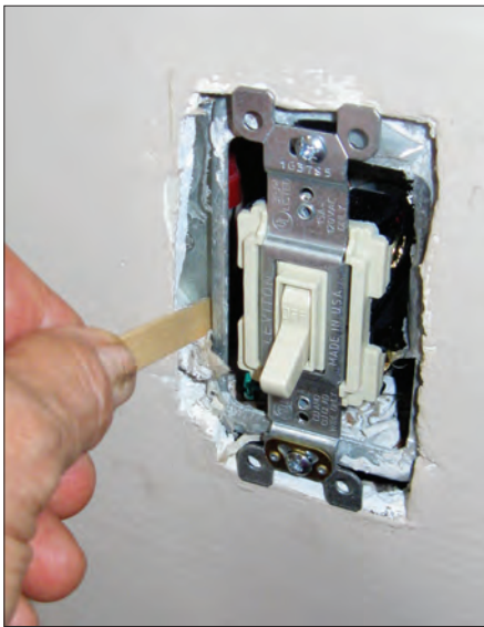
Turn off the circuit breaker and use a nonconducting item to check for a leaky gap.
