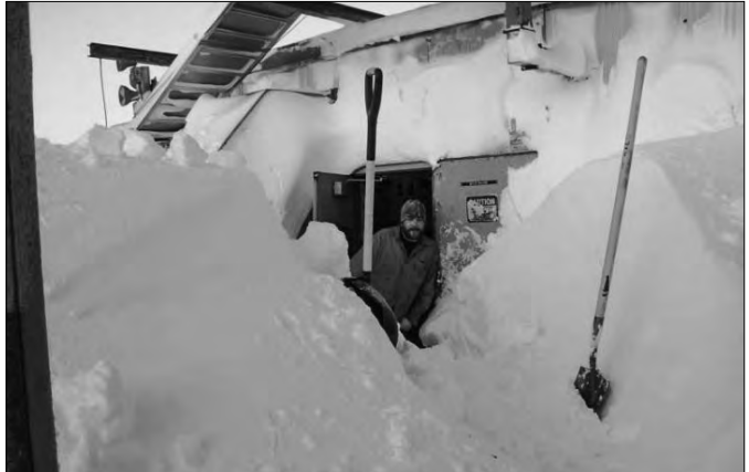
Jud Billing digs out the entrance at AVEC’s power plant in Hooper Bay after a storm.
