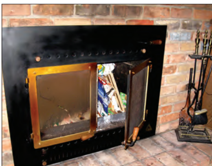
This fireplace draws in outdoor air to improve heated air circulation.
