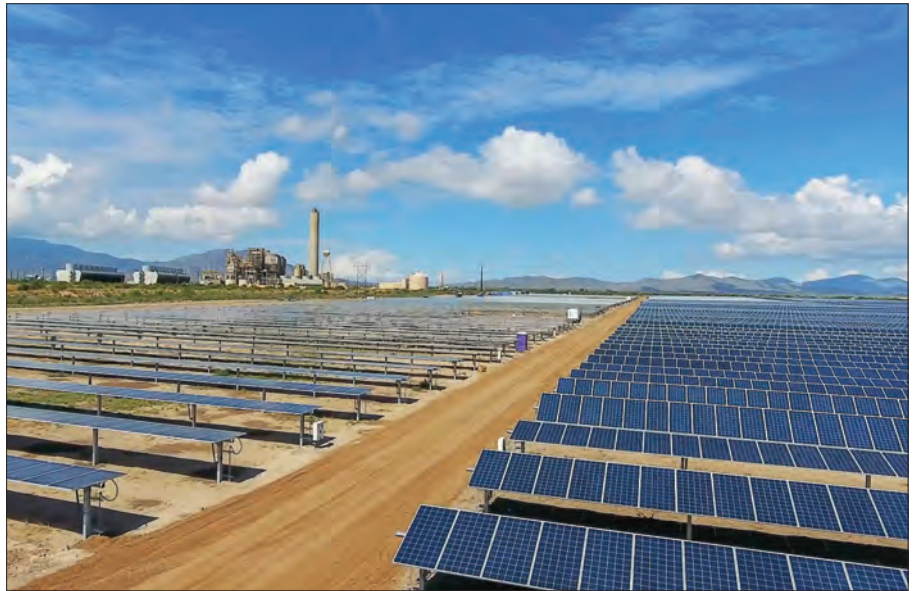
When the 20 MW Apache Solar Project in Cochise County, Arizona, was dedicated September 22, 2017, Congresswoman Martha McSally (AZ-CD2) called it a great example of a renewable energy project done right. “This is a great example of a bottom-up, community-driven investment in innovation, and a community-driven commitment to energy diversity, as opposed to a top-down decision made by bureaucrats in Washington, D.C., telling everybody what to do in a ‘one size fits all’ way,” McSally said.
