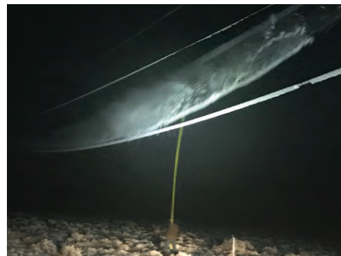
Ice falls in sheets and wires spring back after a lineman uses an insulated "hot stick" to knock ice off the power line. See more ice-storm photos on page 28.
