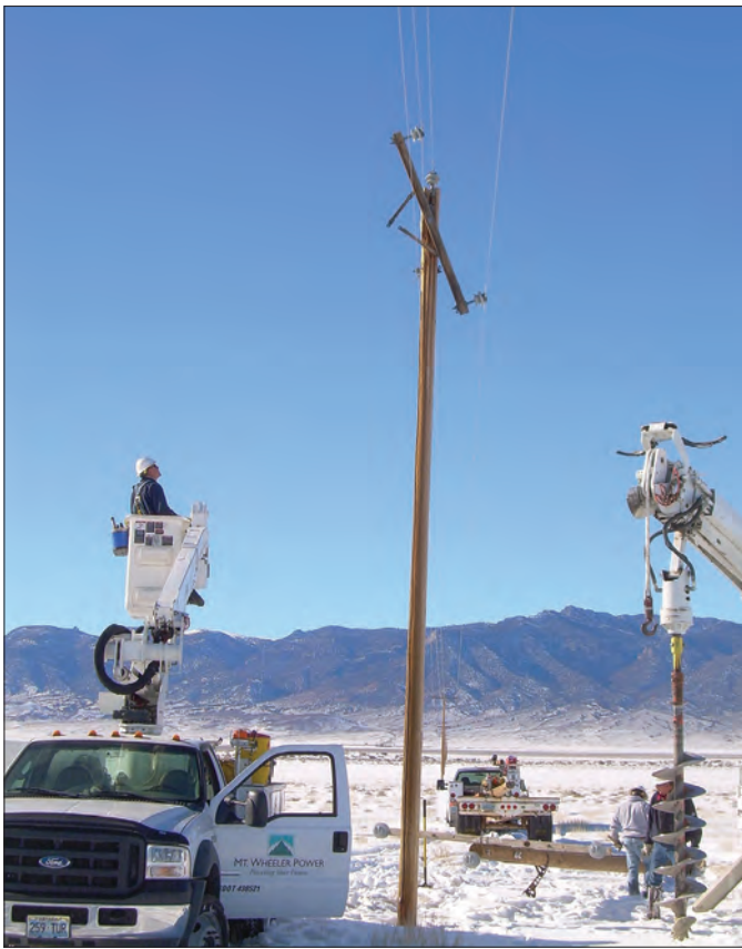
Heavy snow on power lines can cause poles to snap.
