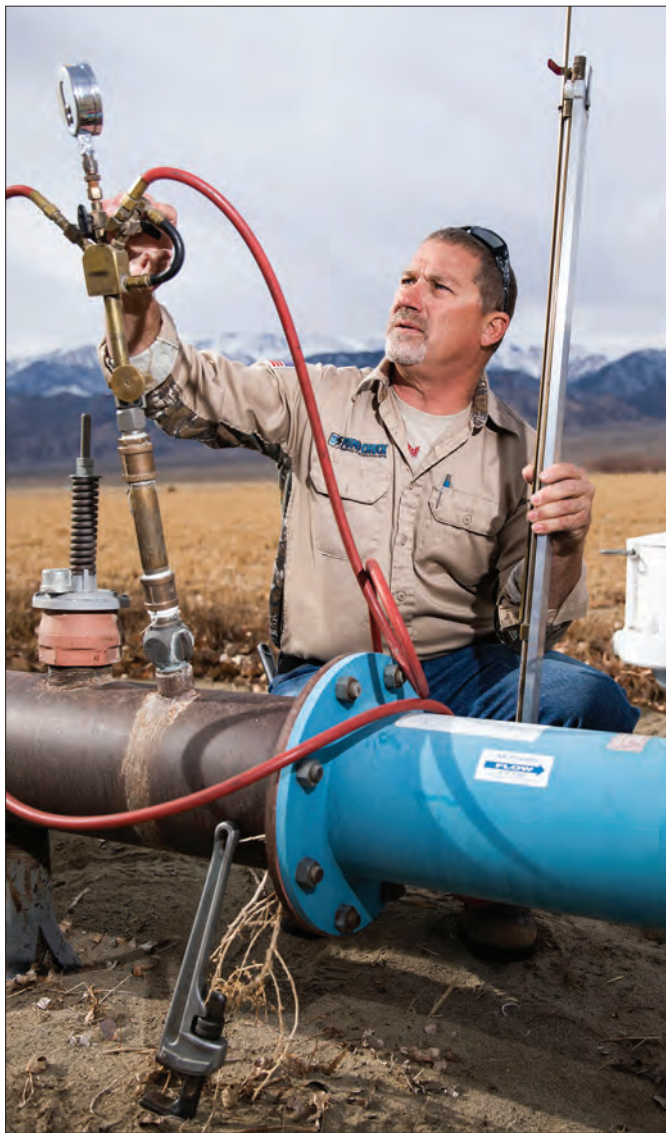
Electrician Jon Lee works on a pitot tube and a manometer, which measure water flow and pressure as he tests the efficiency of a pump in Esmeralda County. Lee was one of the speakers at the 2019 Irrigators Meeting at the Dyer Community Center.
