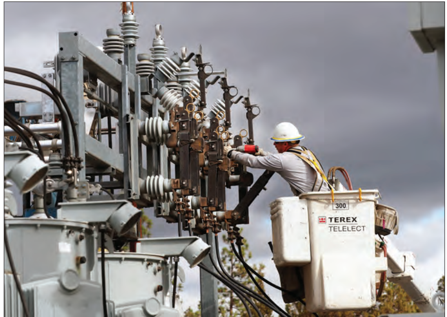
Last year's expansion work at the Sisters Substation by CEC lineman Boone Wagner is an example of the kind of project needing capital investment during the next 10 years.
