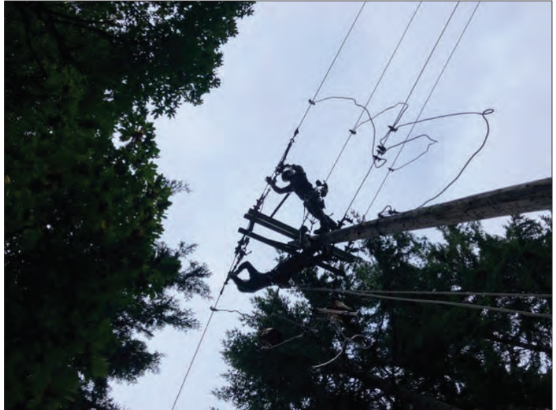
Above, Foreman Brad Jarmain's crew replaces a pole on Reservoir Road, near CPI's Philomath office. Above left, Foreman Aric Williamson's crew performs work in the Harrisburg area as part of the 2018 system improvement plan.
