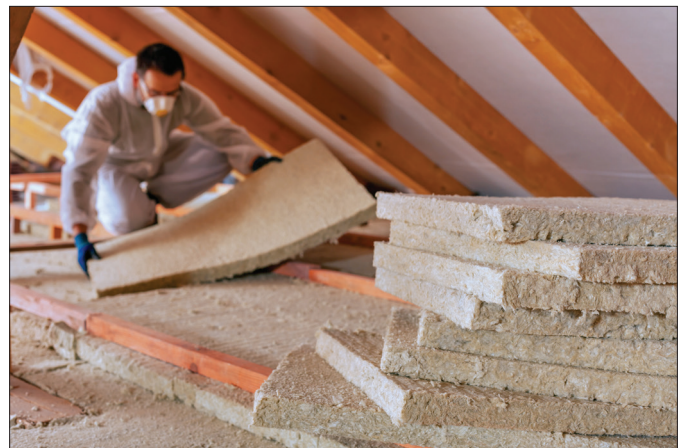
Install insulation in the attic and caulk around windows to make your home more energy efficient.
