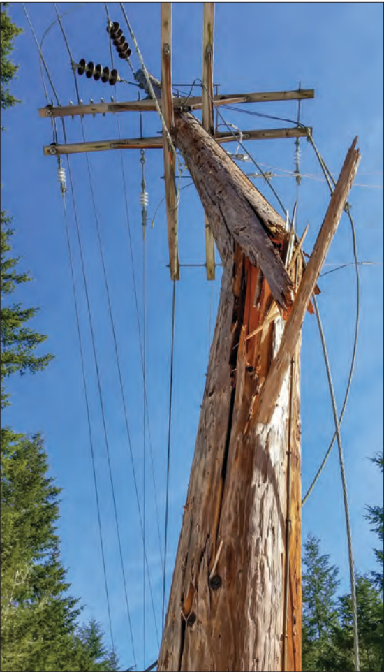
A broken pole carrying both transmission and distribution lines complicated the repair. Photo by Matt Yates
