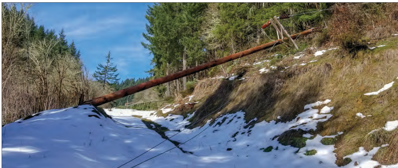
One of many broken transmission poles litters a right-of-way west of Elkton.
