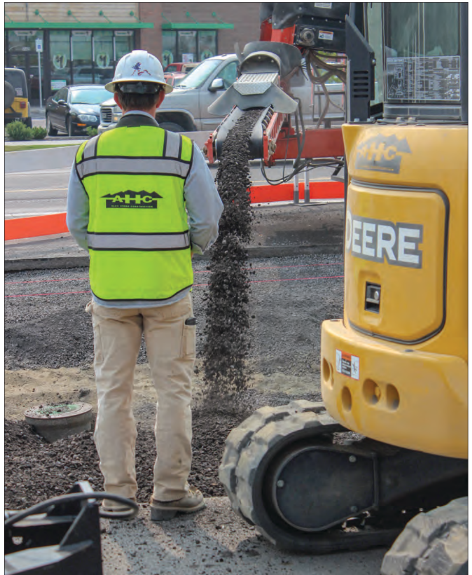
A bed of gravel is laid down before concrete is poured, giving the west side of Highway 97 through La Pine a new sidewalk. The beautification project includes new overhead lights, crosswalks with flashing beacons, landscaping and new pavement.
