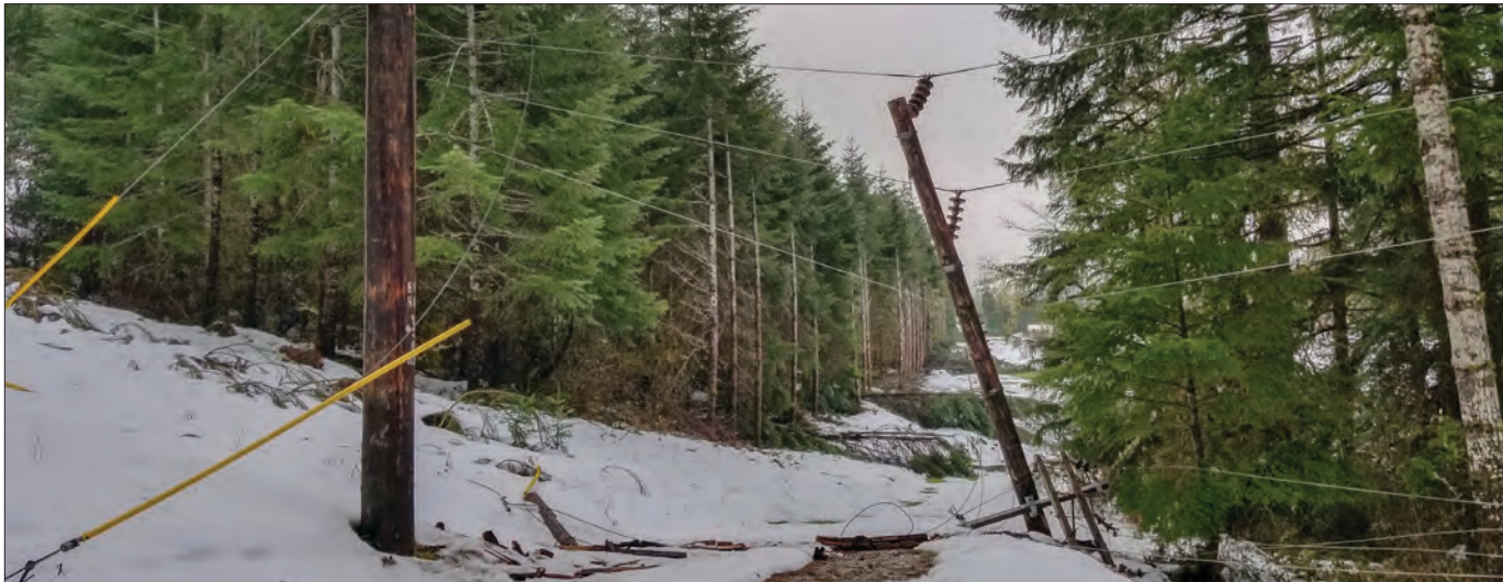
Structures with both transmission and distribution lines were brought down during the late February storm. Photo by Matt Yates
