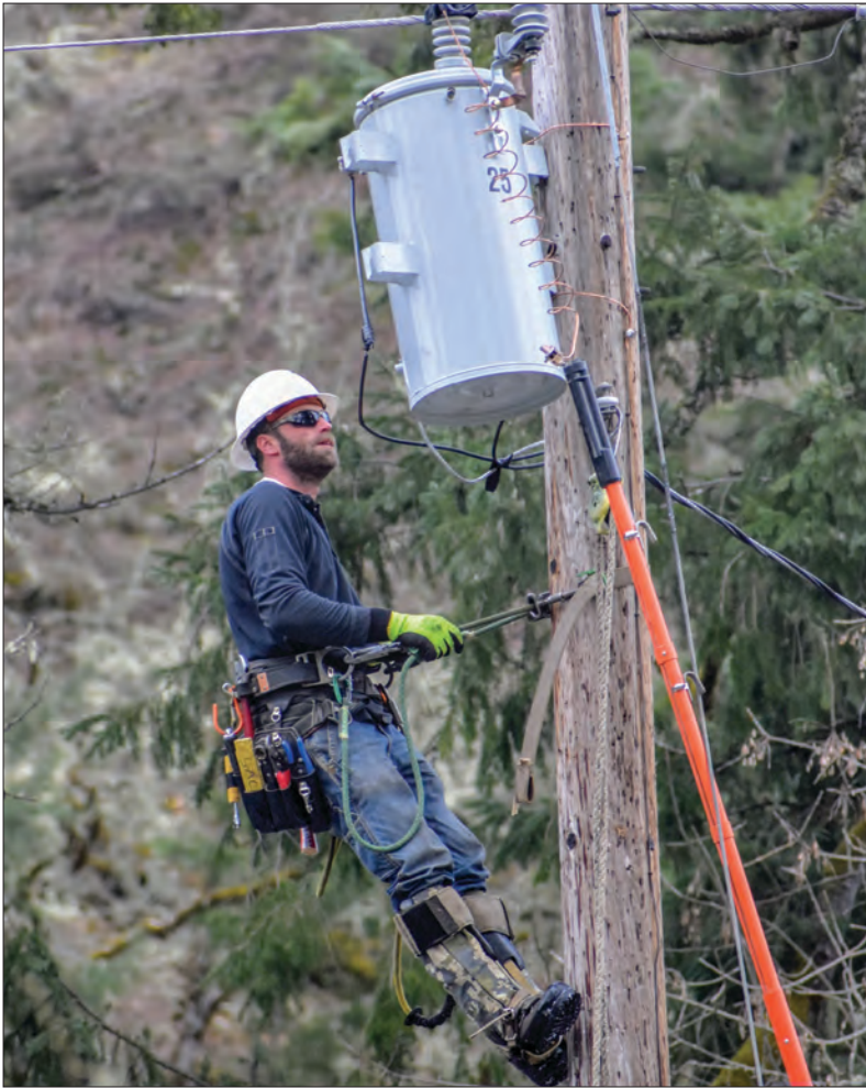
Apprentice Lineman Jeremy Sackett checks a transformer for damage. Photo by Joy McMullin
