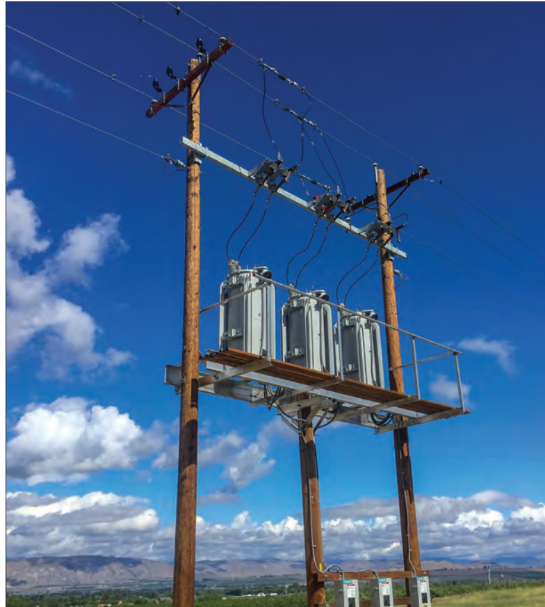
Wood power poles are still the most common.
