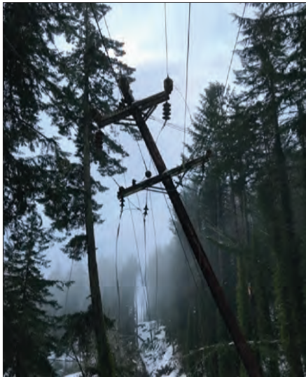
Fallen trees over power lines caused many outages in difficult-to-reach areas.
