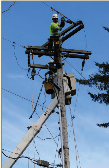
The Tillamook PUD basic charge covers the cost of making power available to every customer including putting up the poles and wires that carry the power to your homes and businesses. Apprentice Lineman Brandon Oldenkamp, top, and Journeyman Lineman Simon Hagerty string conductor.
