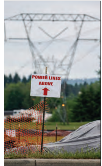
Be alert to the presence of overhead power lines.
