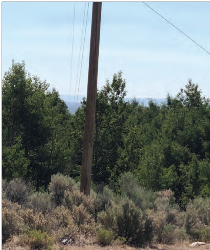
Many WREC poles and power lines—such as the one pictured above—run through areas with heavy brush and thick trees.
