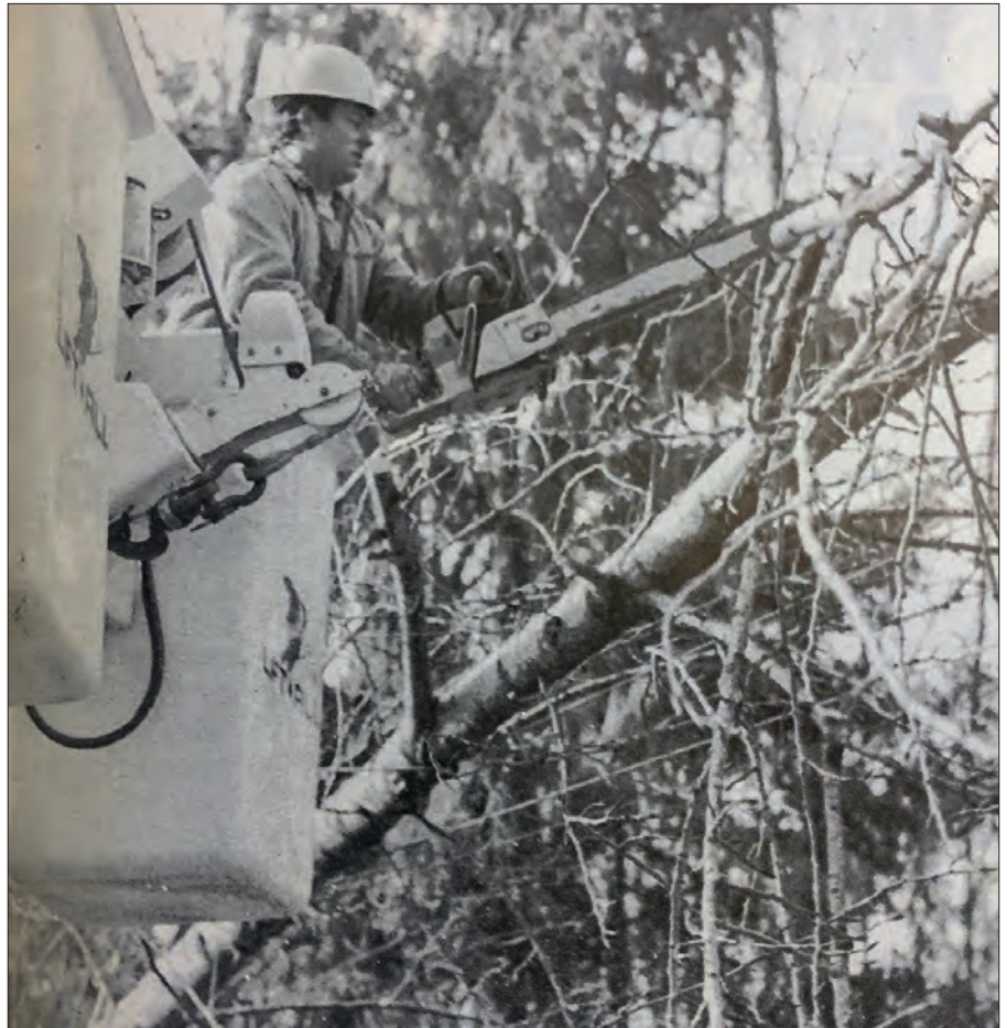
A lineman clears debris from a power line following the Inaugural Day Storm of 1993.
