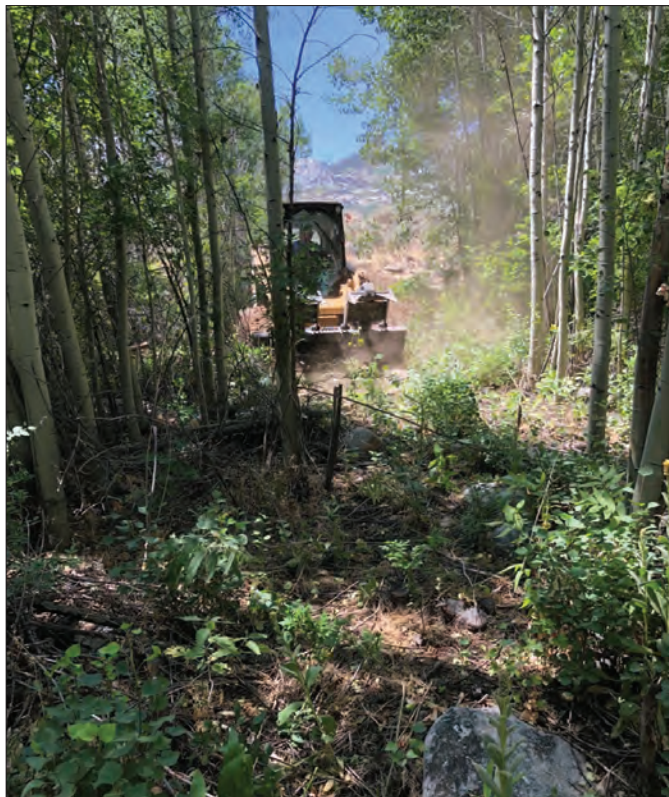
While maintenance projects can be time-consuming and require heavy equipment, clearing brush from around poles is a vital part of protecting equipment from wildfires.
