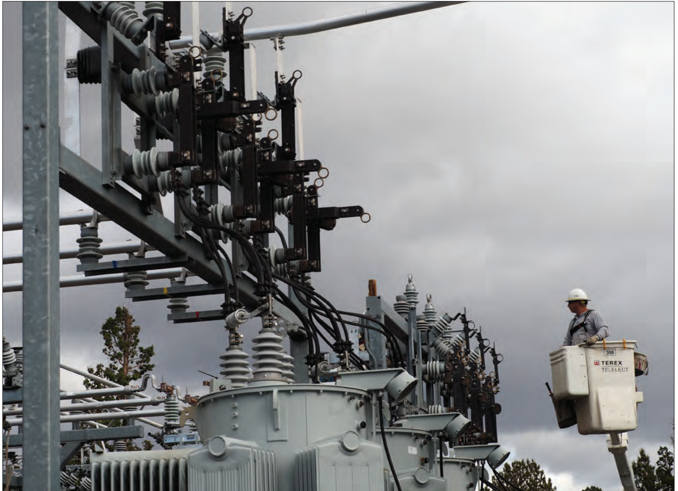
Substation upgrades are needed to meet the growing needs of CEC members. Photo by Jeff Beaman
