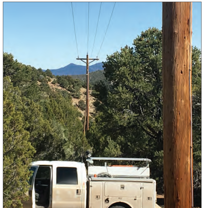
While maintenance projects can be time-consuming and require heavy equipment, clearing brush from around poles is a vital part of protecting equipment from wildfires.
