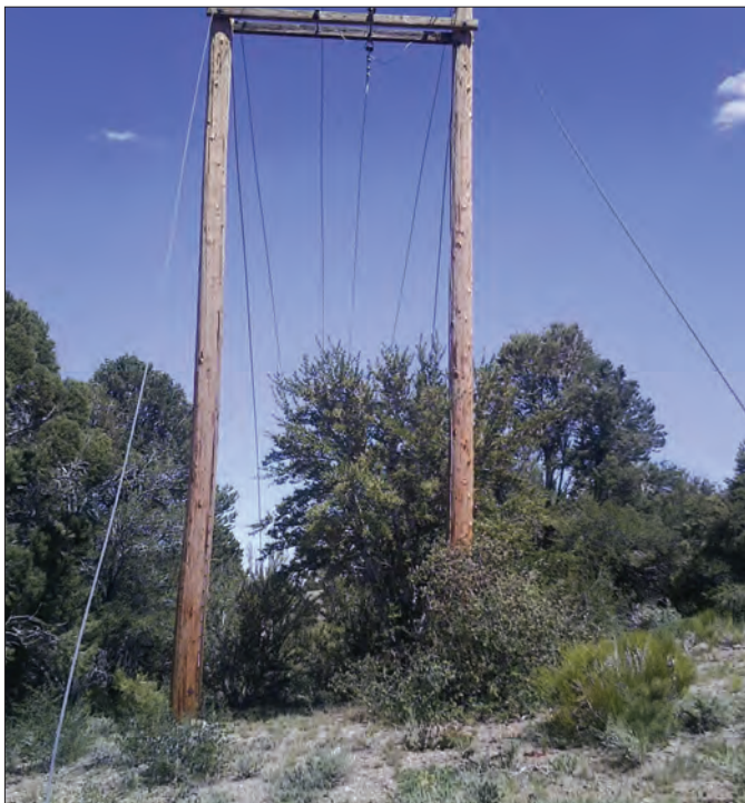
Many Mt. Wheeler Power poles and lines—such as those pictured above—run through areas with heavy brush and thick trees.
