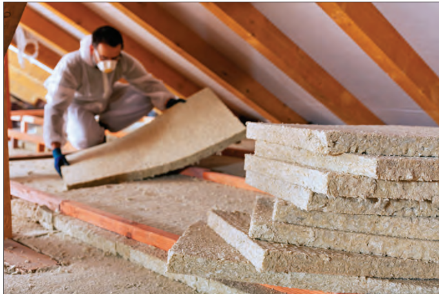
Adding more insulation to the attic can improve the comfort of your home and save on your energy bill.
