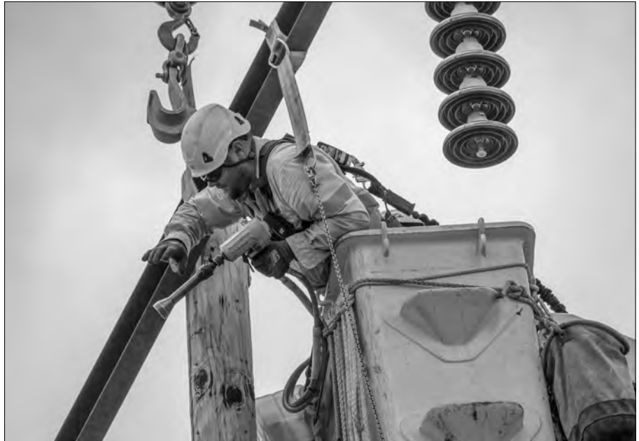
A BPA transmission line crew replaces components on a 230-kilovolt line that was identified as having a high potential for igniting a fire if the equipment failed.
