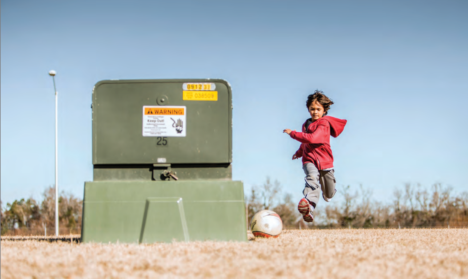
Warn youngsters not to play around or climb on the green transformer boxes that house underground electrical facilities.
