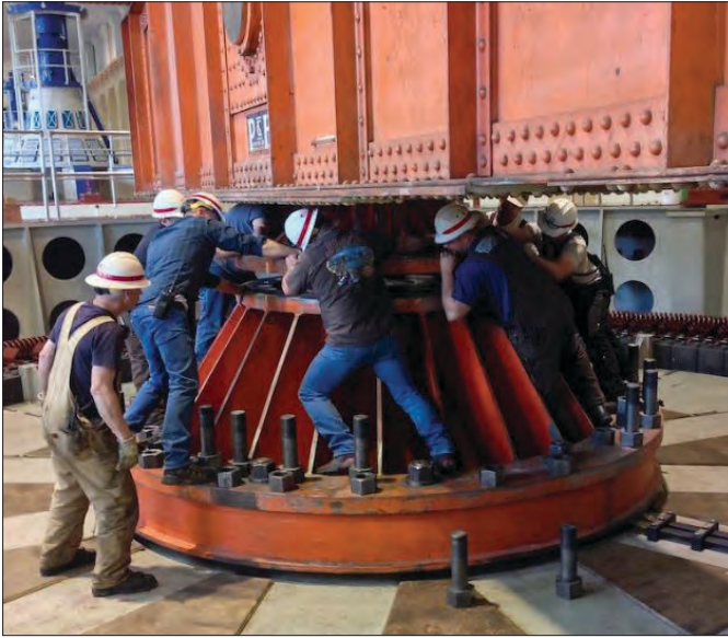
Riggers and mechanics attach a lifting device for a generator at Bonneville Dam.
