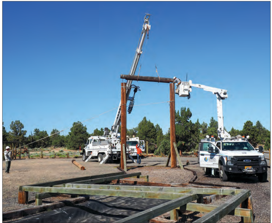
Lineman Grant Young works to remove the top piece of a climbing structure at OYCP.
