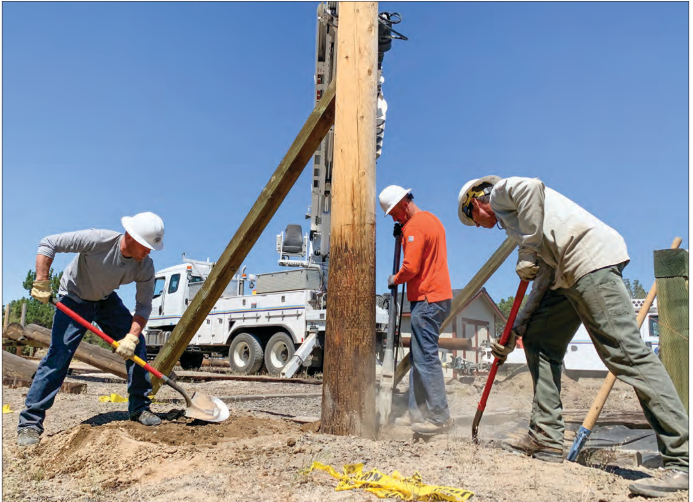
From left, Central Electric Cooperative linemen Grant Young and Rob Lane and Line Foreman Andy Burford set a pole at the Oregon Youth Challenge Program.
