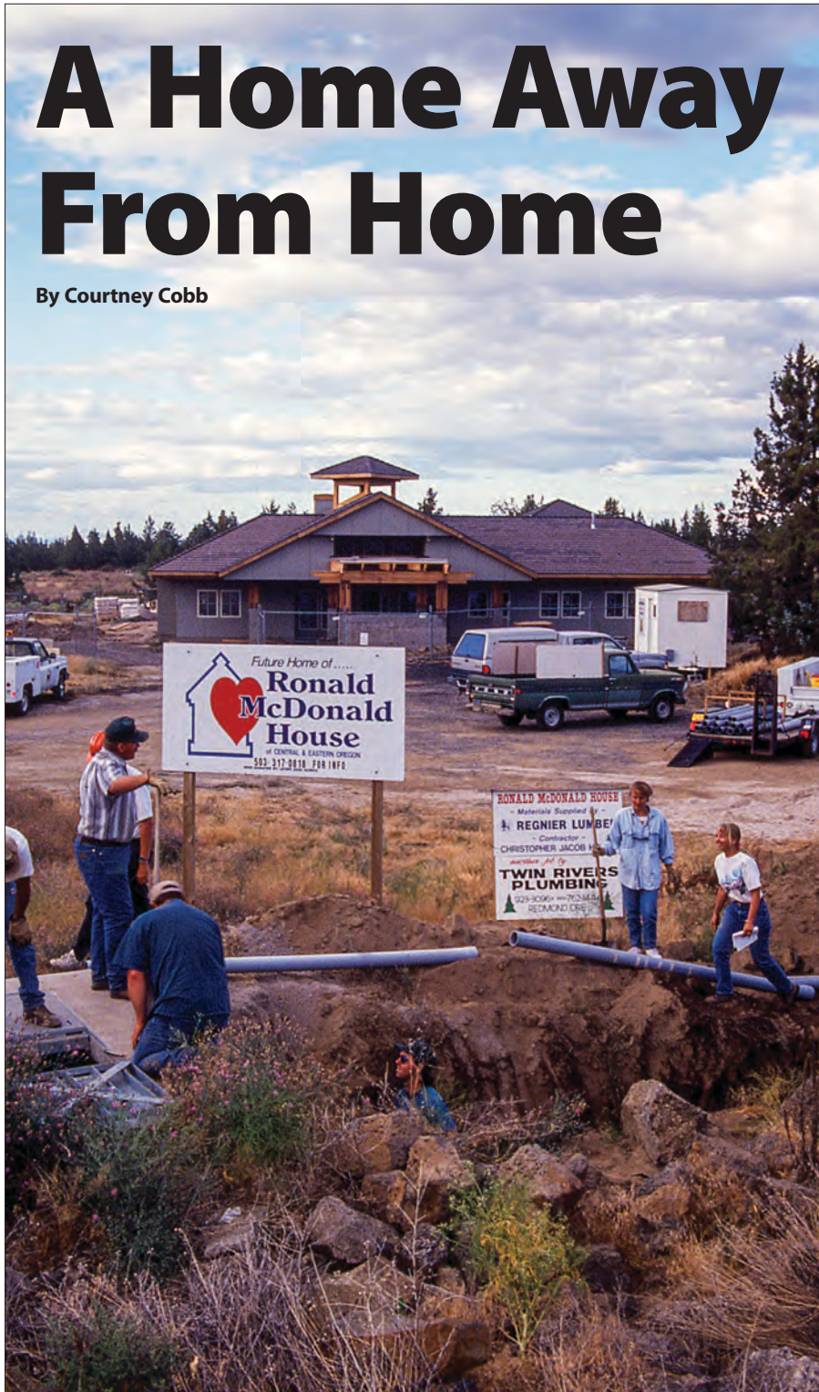
Central Electric Cooperative employees dig a trench for the electrical line to service the Ronald McDonald House built in Bend in 1995.
