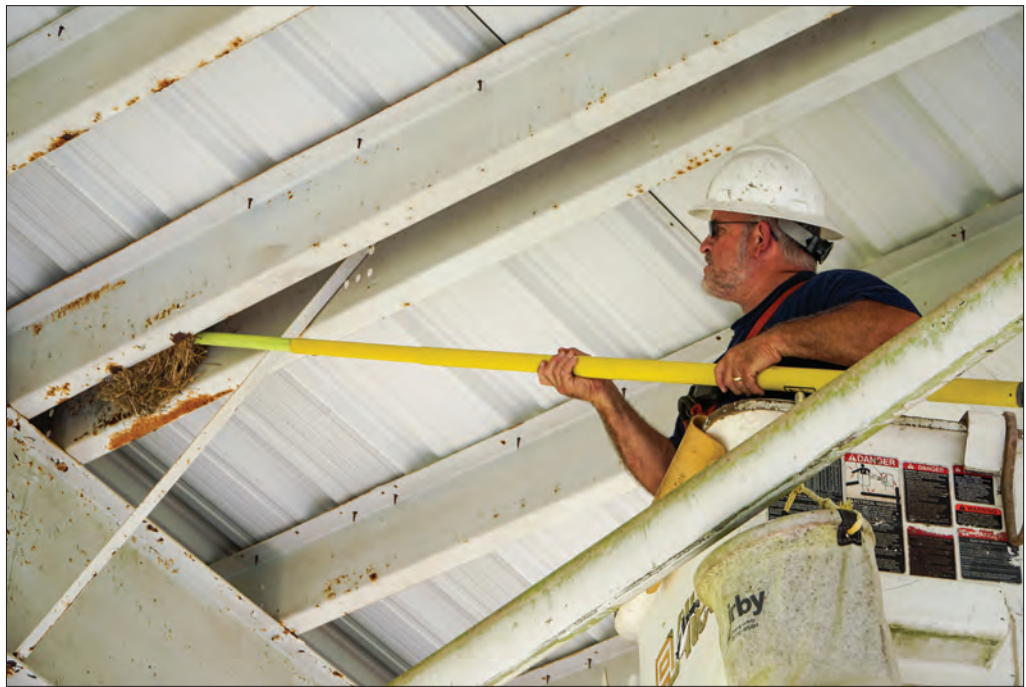
Right before the start of a new school year, EREC Lineman David Greene worked from a bucket truck to remove an empty nest from rafters at an outdoor pavilion used by Bratt Elementary students for physical education classes. Birds leave droppings on the concrete and occasionally knock down straw from the nests.
