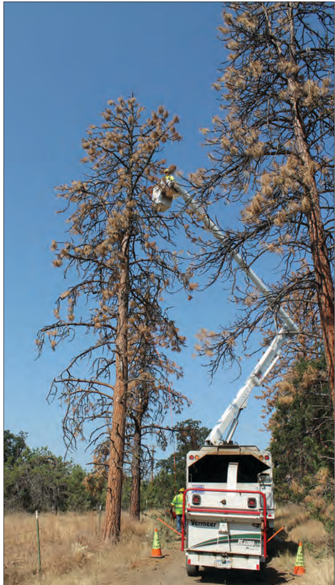
Above, contractor crew Trees LLC ropes off a hazardous tree at the top to safely fall it away from Wasco Electric Cooperative's three-phase line in the Wamic area. Above left, a fallen hazardous tree shows disease.
