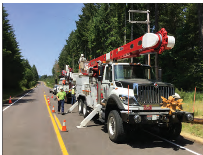
Above, Blachly-Lane crews replace a pole with a unique side arm design. Photo by Matt Smith. Opposite page, crews make Alderwood Substation improvements. Photo by Jeff Jones
