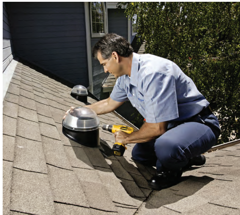
A tubular skylight is installed on a shingle roof. Notice how the shingles fit over the flashing to eliminate leaks.
