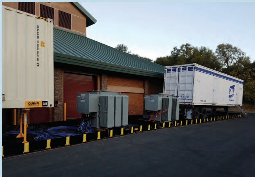
PG&E transported two 1.5-MW backup generators several hundred miles to Placer County, at no charge, enabling the water agency to continue pumping water during a PPS in October. Photo courtesy of Placer County Water Agency
