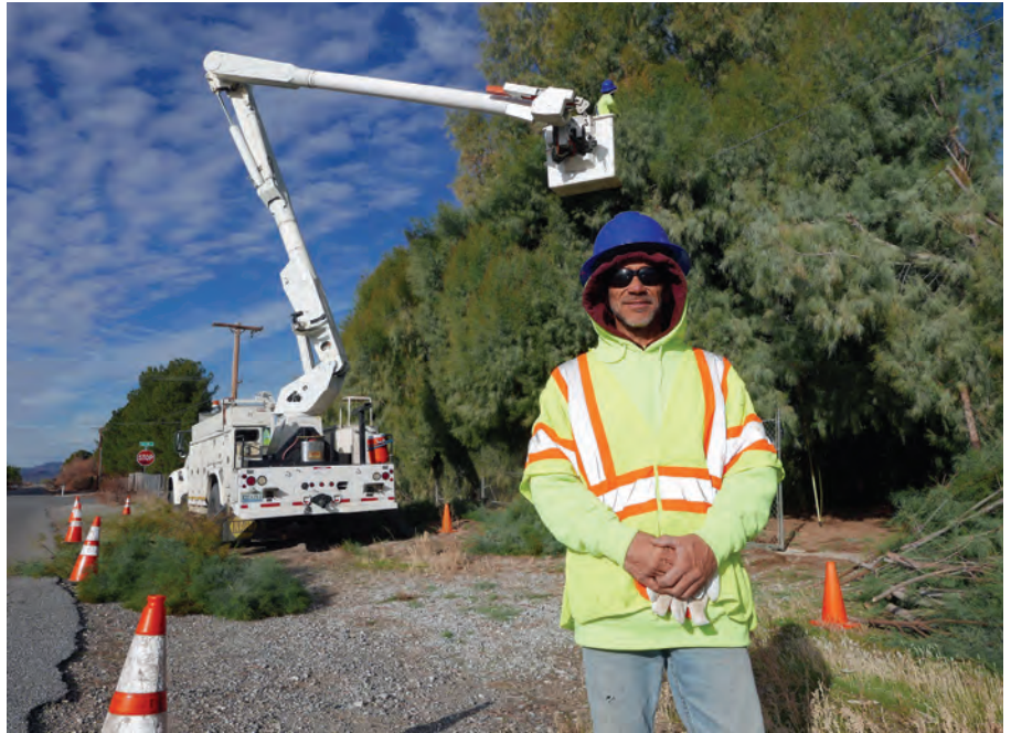
Keith Layton near one of his trucks as a crew clears tree growth from a distribution line near Betty Avenue and North David Street in Pahrump. VALLEY ELECTRIC PHOTO
