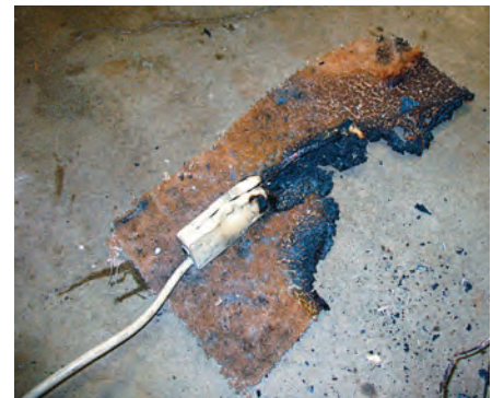
A failed power strip sparked a fire that caused an estimated $5,000 damage to a home. Use multi-outlet devices sparingly. If you need more outlets, hire an electrician. PHOTO COURTESY OF TUALATIN VALLEY FIRE
