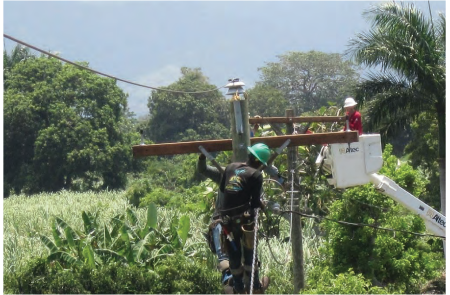
Linemen from Texas work to extend distribution lines to new service territory in Haiti PHOTO COURTESY OF TRINITY VALLEY ELECTRIC COOPERATIVE
