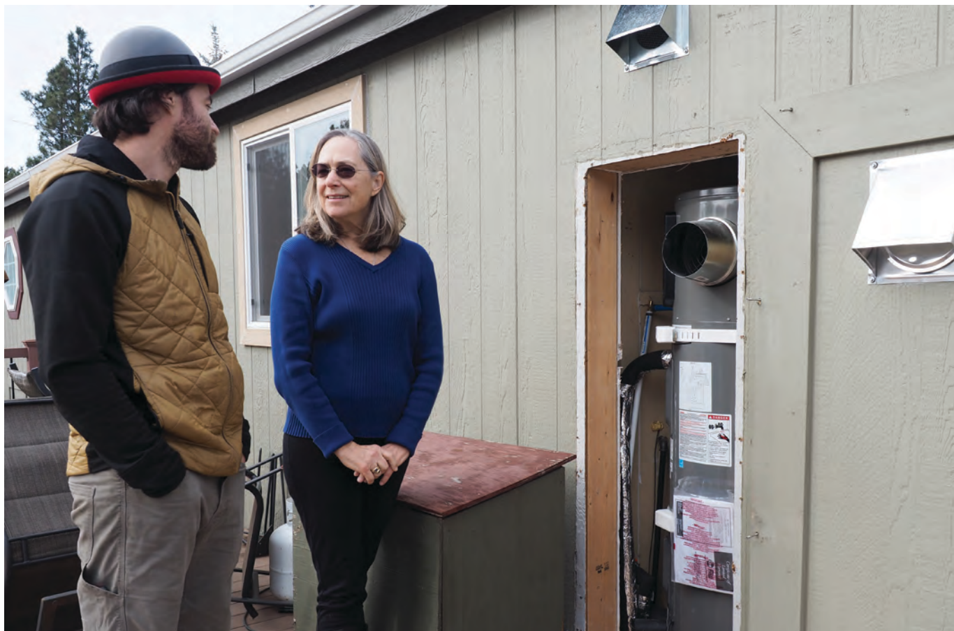
Randi Schuyler talks with her son Lebn Lovejoy about the installation of her energy-saving heat pump water heater.
