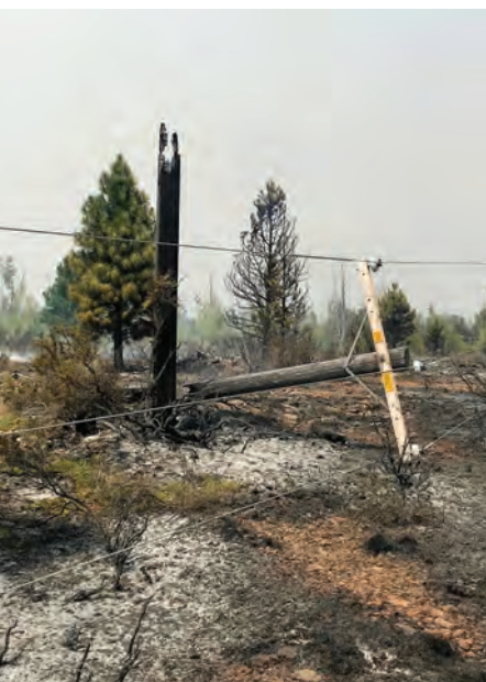
A 2018 wildfire destroyed the electric distribution system serving Eagle Lake in Northern California, leaving about 1,000 people without power. PHOTO COURTESY OF LASSEN MUNICIPAL UTILITY DISTRICT
