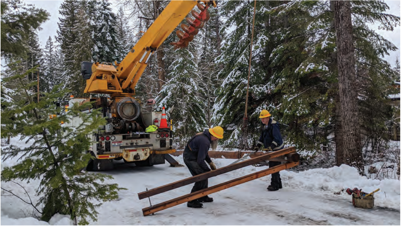
NLI linemen prepare to install a power pole. PHOTO BY KRISTIN METTKE
