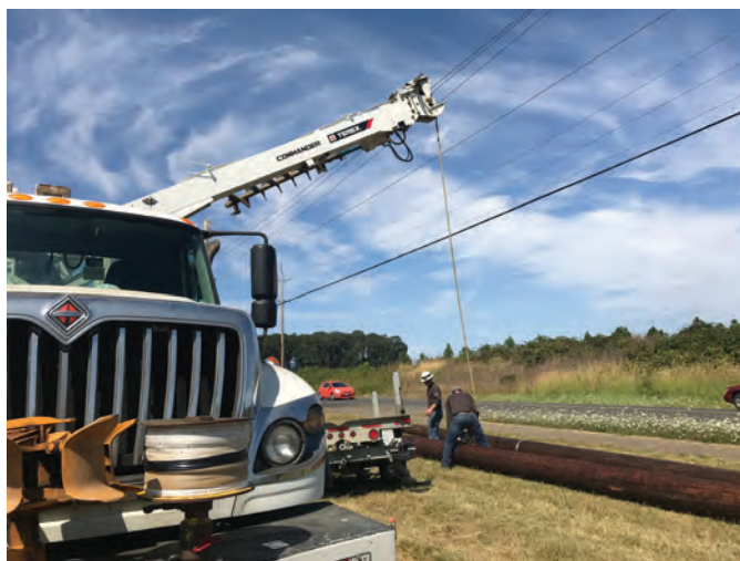
ABOVE: Brad and crews use a derrick digger to set new poles. TOP: Getting to an outage isn't always as simple as driving down the road.
