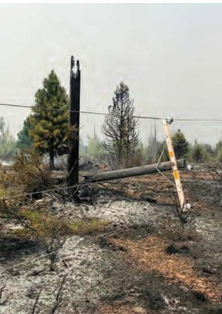
A 2018 wildfire destroyed the electric distribution system serving Eagle Lake in Northern California, leaving about 1,000 people without power. PHOTO COURTESY OF LASSEN MUNICIPAL UTILITY DISTRICT
