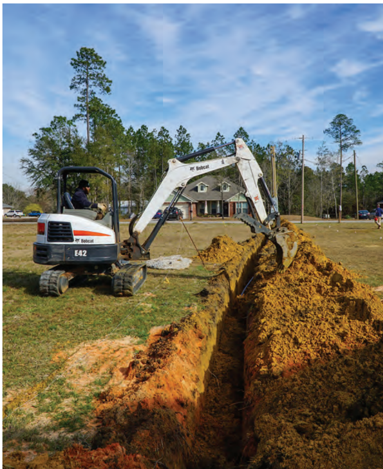
Crews have safety training on the various equipment and machinery they operate, such as the Bobcat Wesley Clark uses to lay underground power lines.
