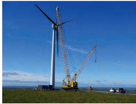
A crane is used to install a new 900-kW turbine in St. Mary's.
