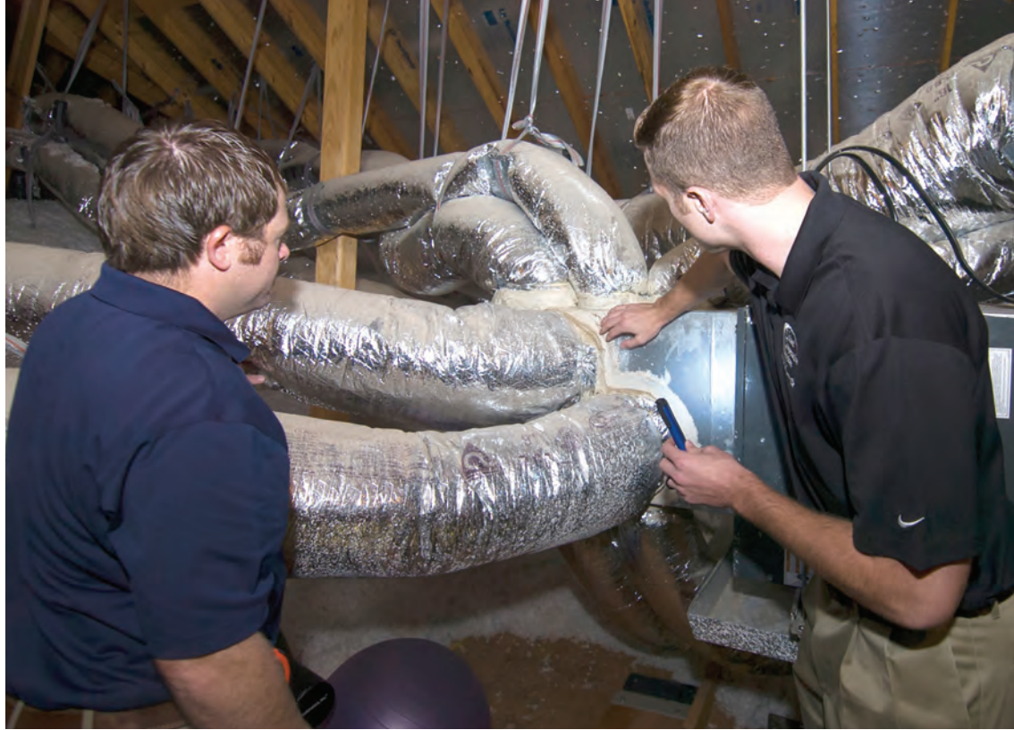
Inspecting and sealing furnace ducts are high-impact projects best left to professionals.
