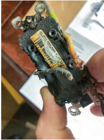
If your lights flicker and you smell burning plastic, call an electrician. This outlet was found thanks to an attentive homeowner.
