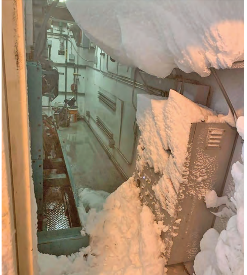
This scene greeted AVEC crews numerous times as they opened the door to this generating module in Savoonga, even though they removed snow every hour. Strong winds blew snow into the module through the intake louvers. The snow built up from the roof to the floor, creating a snow wall near the entrance. Snow covering the Hampton Drive melted and fried some components on the control panel.
