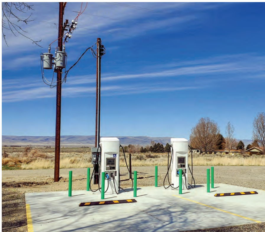
The EV chargers in Orovada are at the Sawtooth Station on Highway 95.
