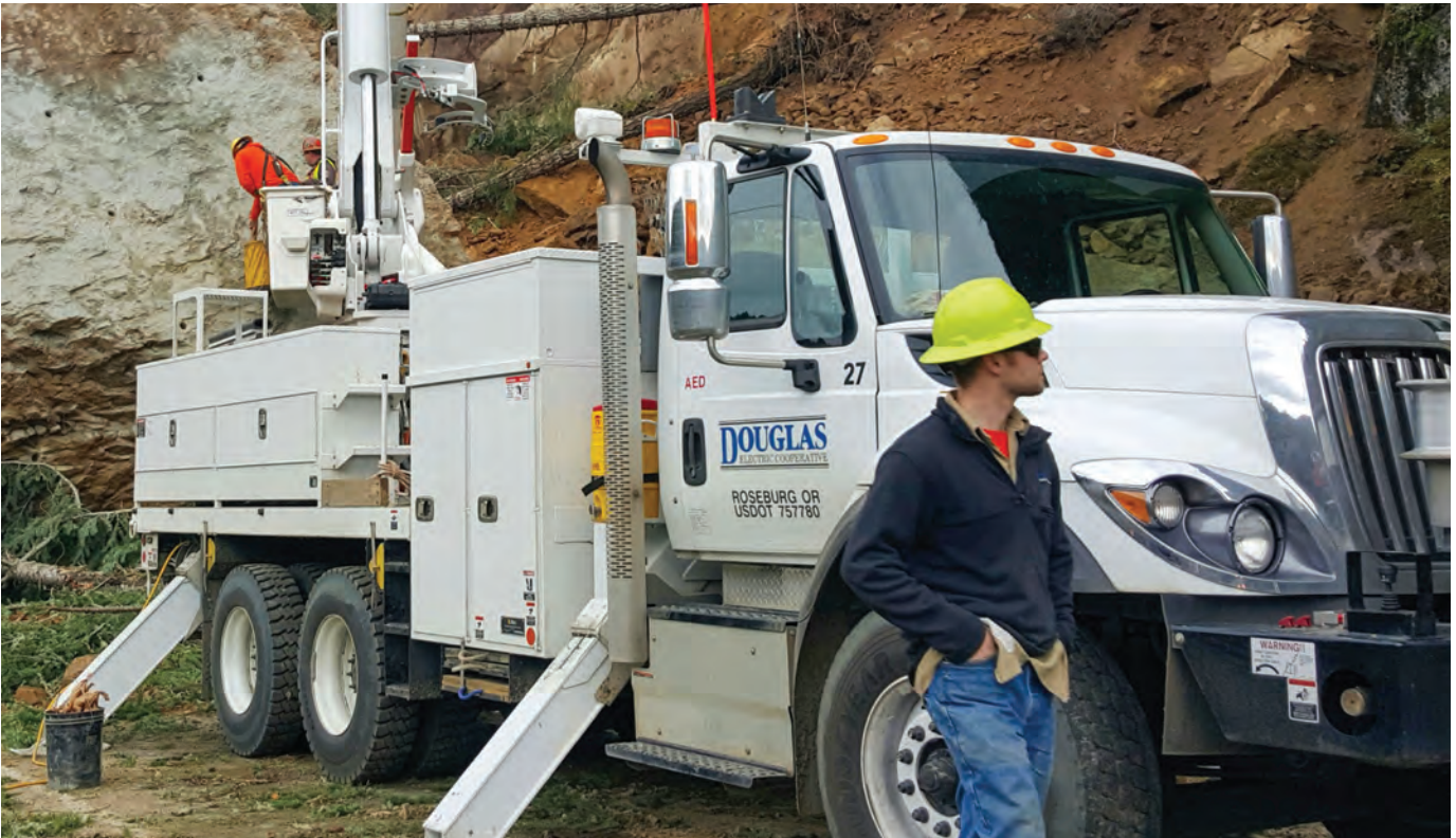
Rockslides and landslides present another hazard for DEC linemen. Slides not only take out power lines, they make access difficult for linemen who are working to get the lines back up and powered.
