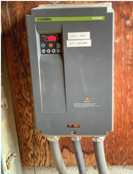
Bierly Acres' variable frequency drive can help save time, energy and water.
