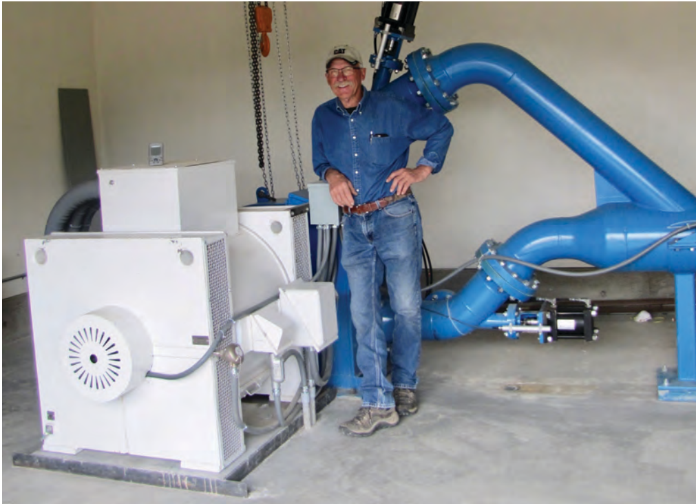
Rock Creek Hydro LLC's Gordon Fulton worked with Salmon River Electric Cooperative to build a new small power plant.
