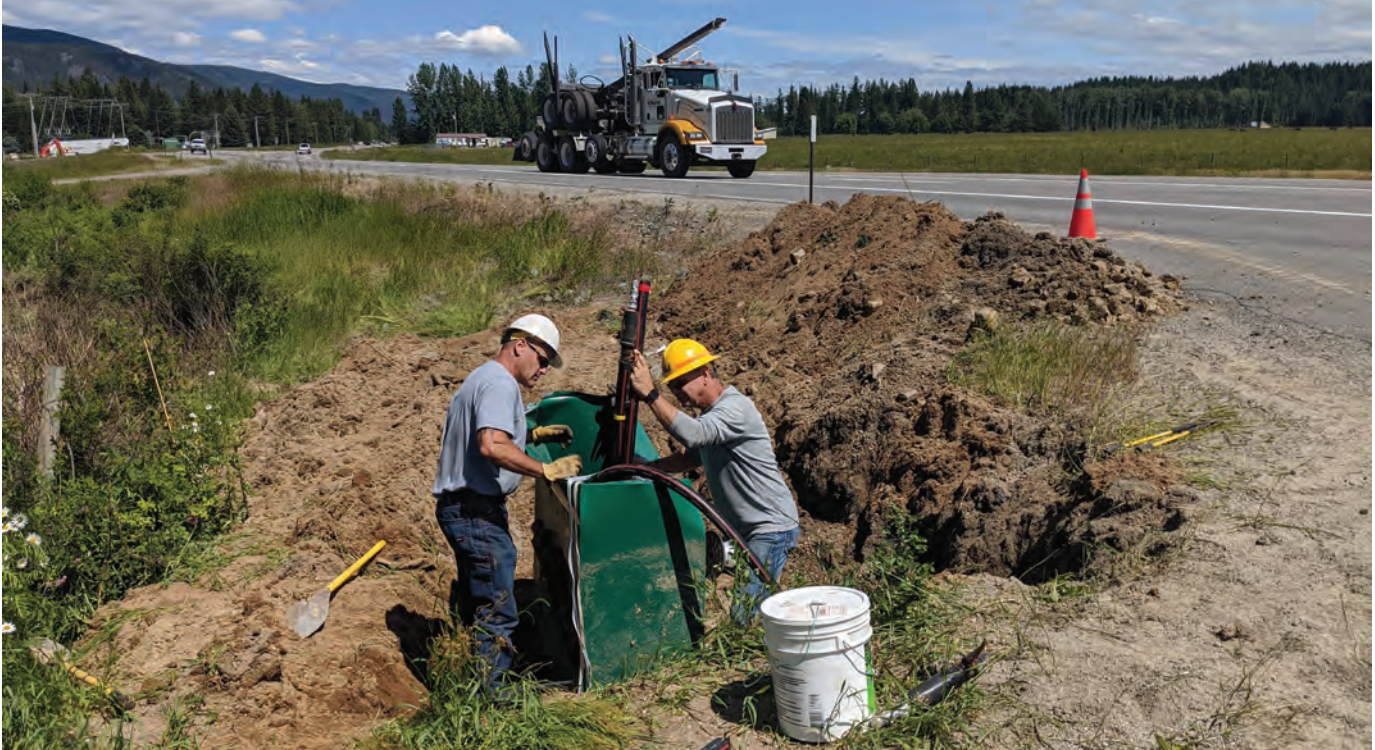
NLI linemen Bill Murray, left, and Marc Hull repair a junction box. Power was rerouted to prevent an extended outage.
