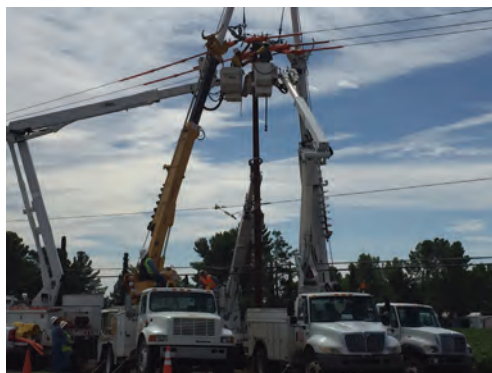
It takes the coordinated effort of linemen to install a new power pole.
