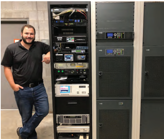
Jordan Tomlinson, 38, stands next to the radio transmitter and equipment rack for KSAS (Kiss-FM) in Boise, Idaho. He says working at the high school radio station motivated him to pursue a career in radio. He is director of engineering for Townsquare Media in Boise, and helps out the high school radio station with equipment and maintenance.
