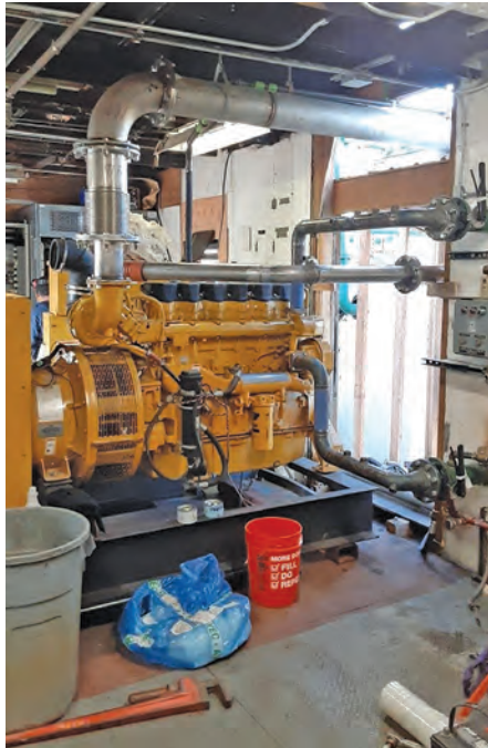
LEFT: One of two Caterpillar 3456 500-kilowatt gensets with marine manifolds awaits installation. PHOTO COURTESY OF AVEC
