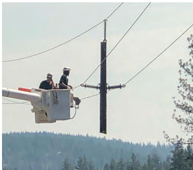
TOP: Crews work 14-hour days to restore power after fire damaged transmission lines and poles. ABOVE: Linemen replace 25 transmission poles.
