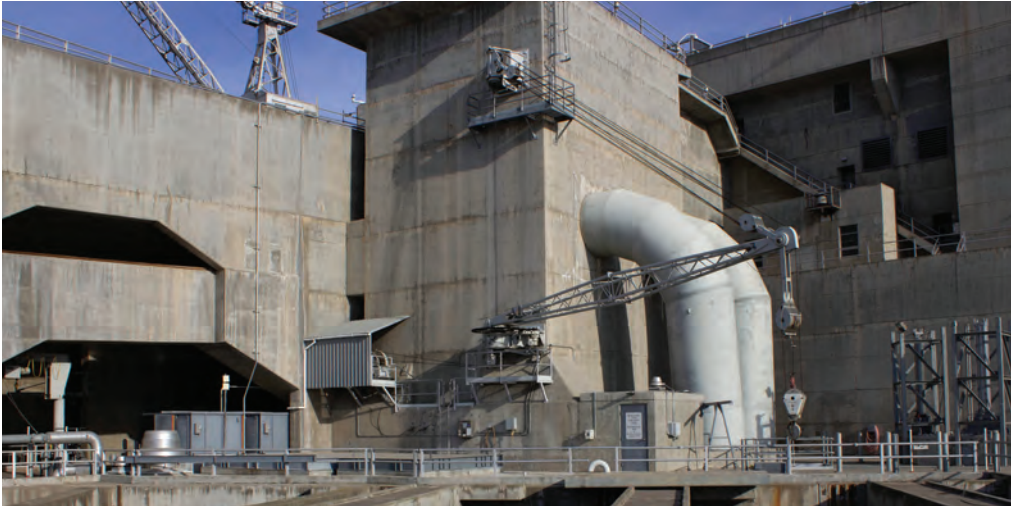
Klickitat PUD and Northern Wasco County PUD opened the McNary Dam Fishway Hydro Project together in the 1990s.
