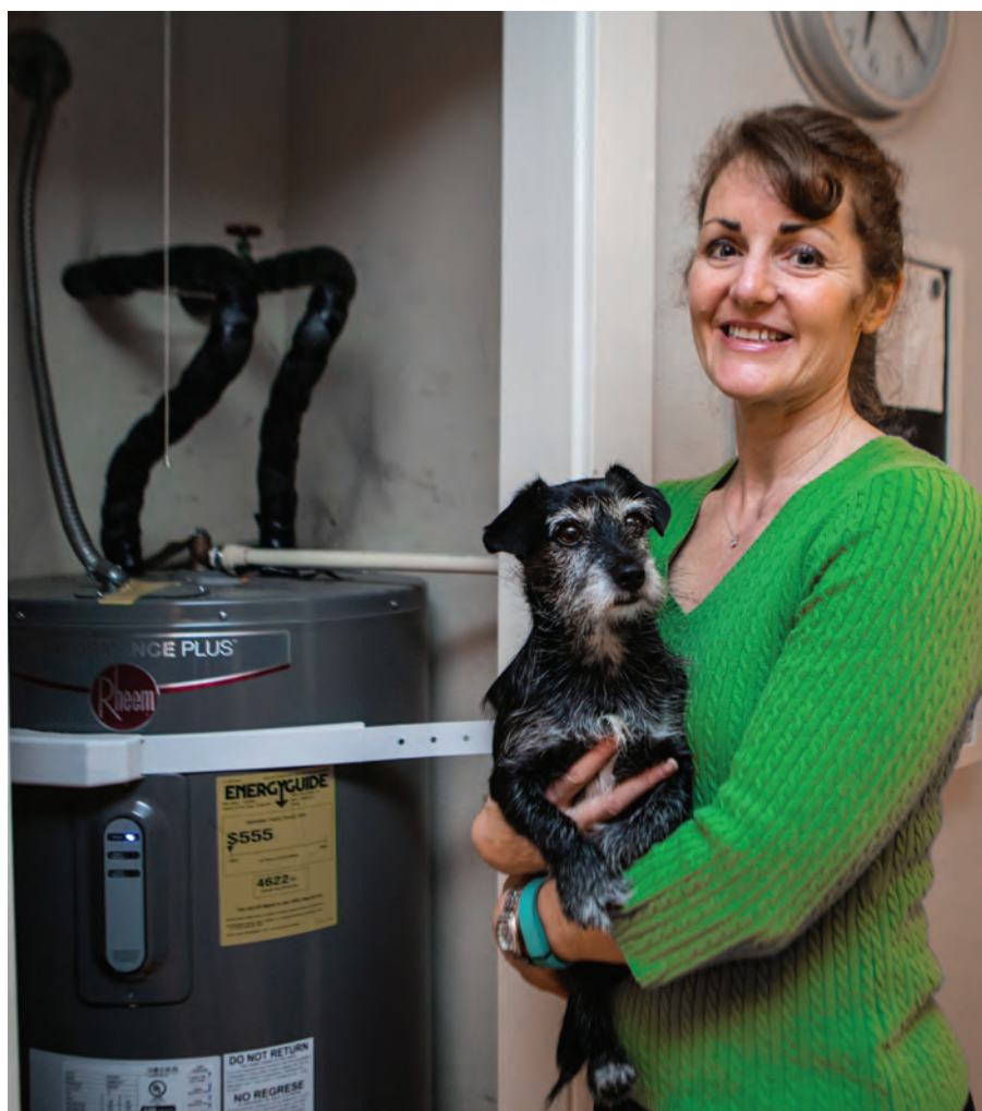
Insulating the first several feet of the hot water pipe where it leaves the tank is an energy saver. PHOTO COURTESY OF MARCELA GARA, RESOURCE MEDIA, EE IMAGE DATABASE
