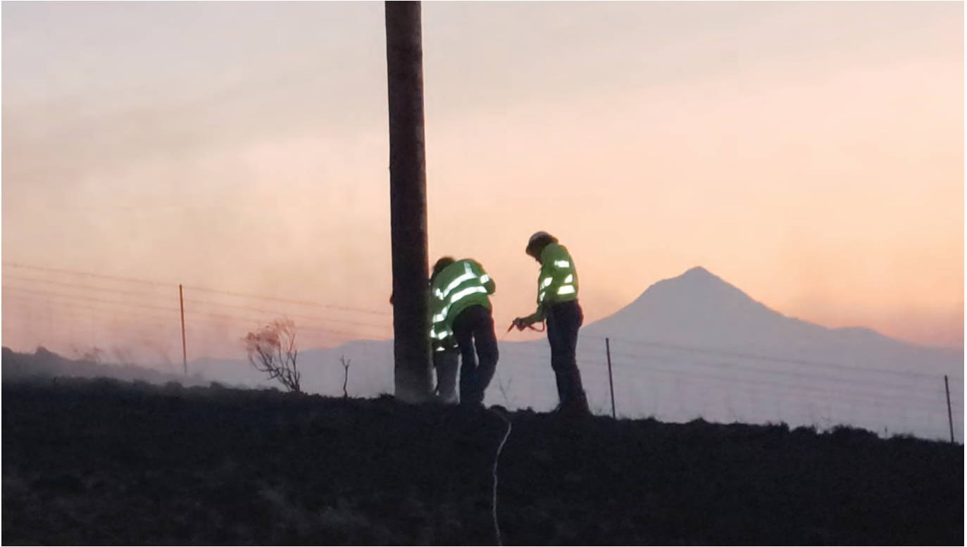
Line crews from Klickitat PUD and Northern Wasco County PUD worked together to restore service after fires damaged the area. PHOTOS COURTESY OF NORTH WASCO COUNTY PUD
