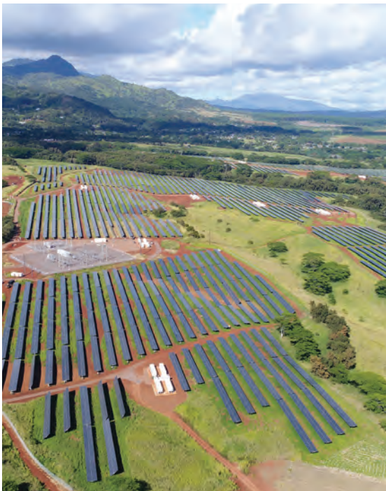
AES Distributed Energy worked with Kaua'i Island Utility Cooperative on the world's largest operational solar-plus-storage system. The 28-megawatt solar plant in Lawai is connected to a 100-megawatt-hour battery energy storage system, providing cheap, clean energy when it is most valuable, instead of just when the sun shines. PHOTO COURTESY OF AES
