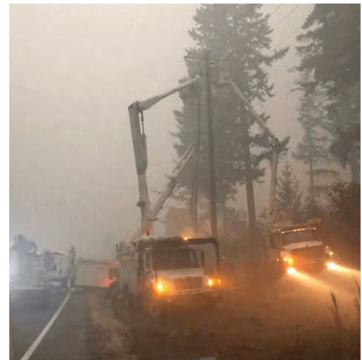
OTEC sent a crew to Marion County to help a fellow co-op repair power amid devastating wildfires. PHOTO BY PAT MCCLUSKEY/OTEC
