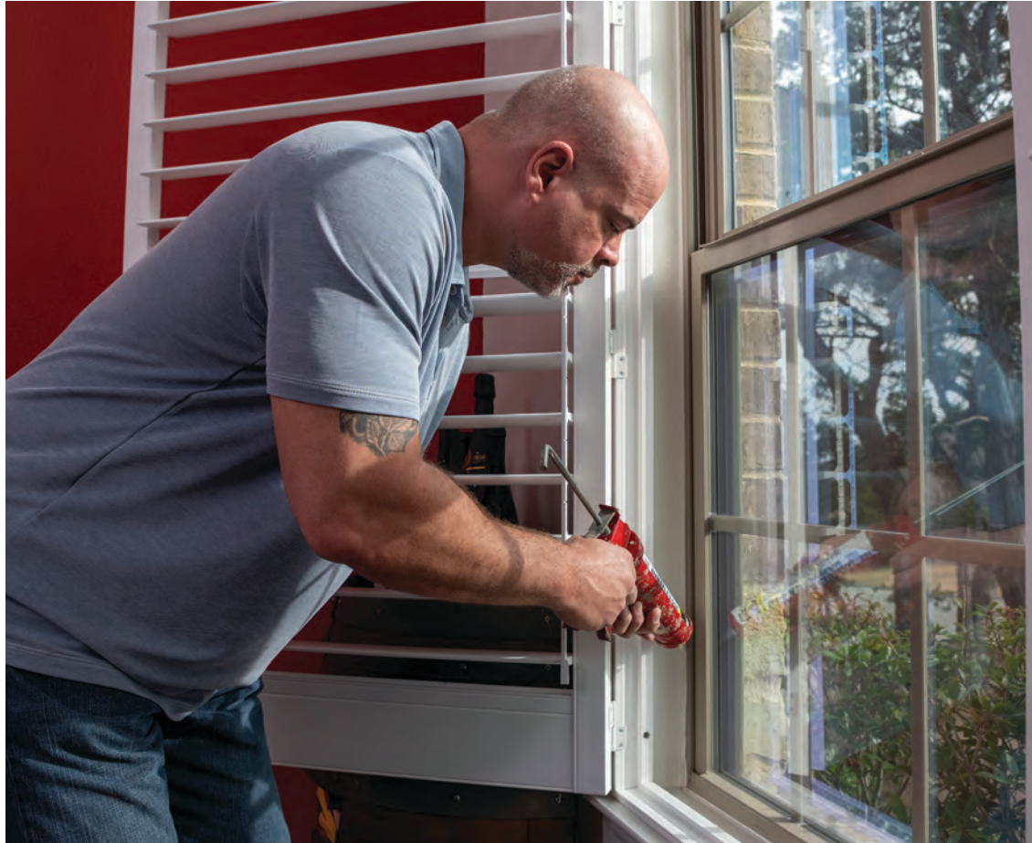
Use caulk to seal gaps around non-moving parts of doors and windows. PHOTO BY SCOTT VAN OSDOL
