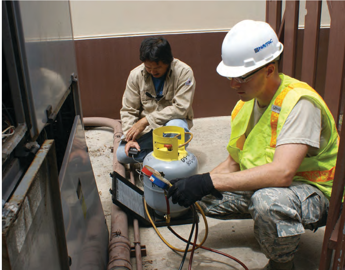
An HVAC professional can inspect and test a furnace to make sure it operates safely and efficiently.
