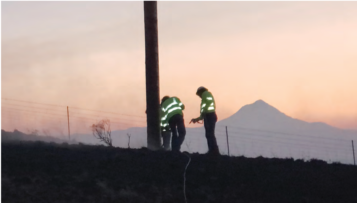
Line crews from Klickitat PUD and Northern Wasco County PUD worked together to restore service after fires damaged the area.
